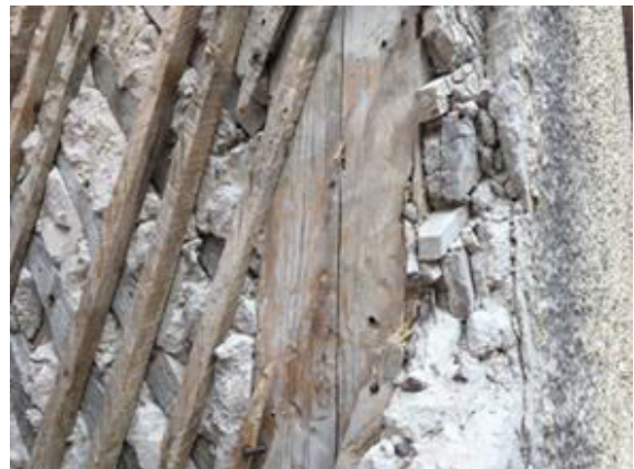
Figure 2. Exposed lime plaster embedded in diagonal wooden slats on another property in Visby. Here the lime and wooden slats were removed in order to apply mineral wool insulation with the goal to improve energy efficiency.
