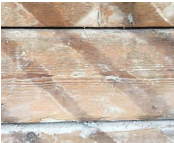
Figure 4. Exposed timber of an historical bole house in Visby (the same property as in Fig. 2 and 3) after the wooden slats and lime plaster had been removed.
